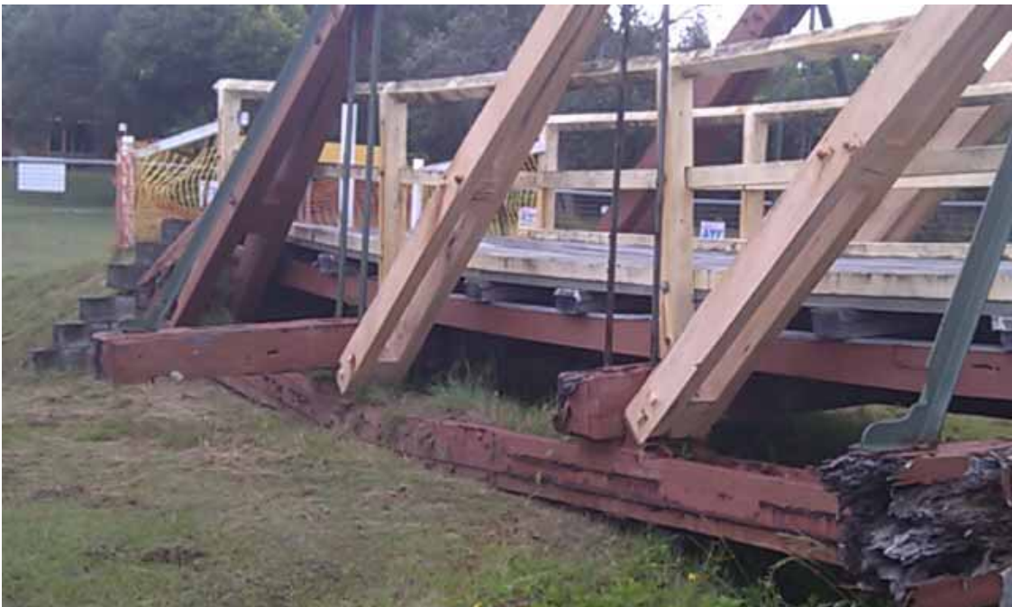
Figure 2 – Deterioration of Girders Story Bridge
