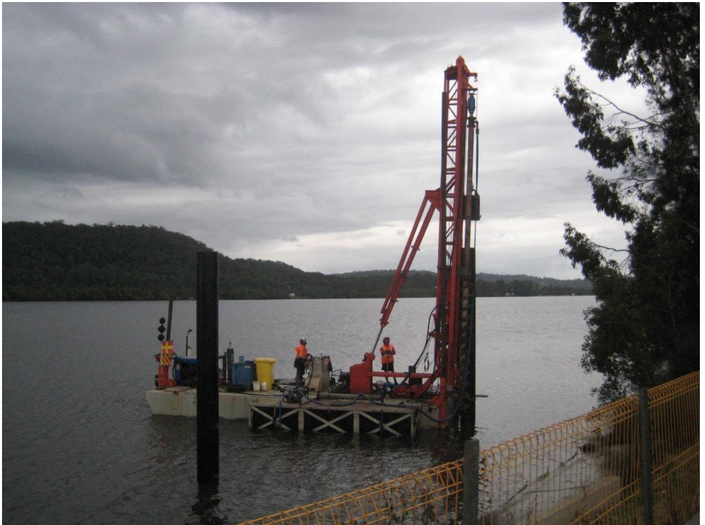
Caption: Work under way this week installing new piles to support pontoons at Maclean's McLachlan Park.
