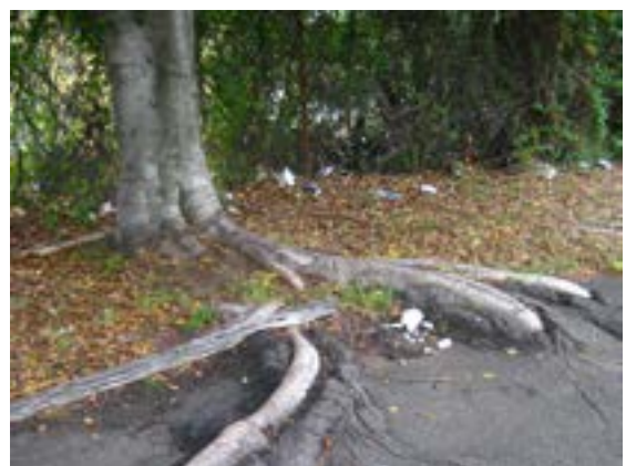
These Ficus microphylla in Rozelle, Sydney have been planted on top of a sandstone escarpment in extremely shallow soil. An inappropriate selection considering the limited soil volume, the roots have severely compromised the footpath.
