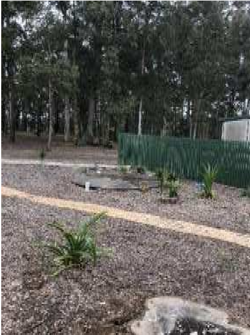
Photograph 1. Amenities septic tank (T1).
