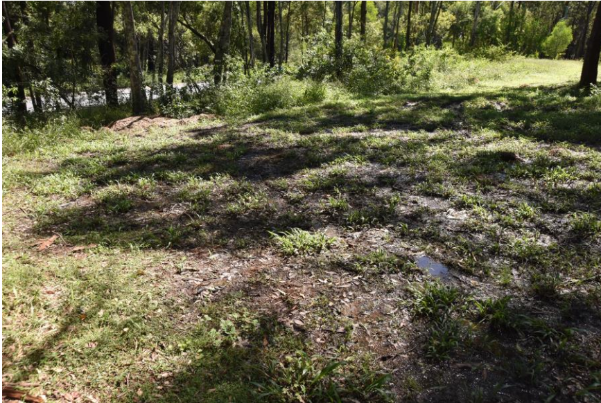
Existing seepage toward old Pacific Highway roadway
