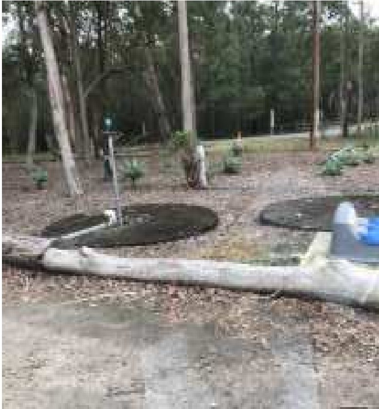
Photograph 6. View of dump point tanks T5 & T6.
