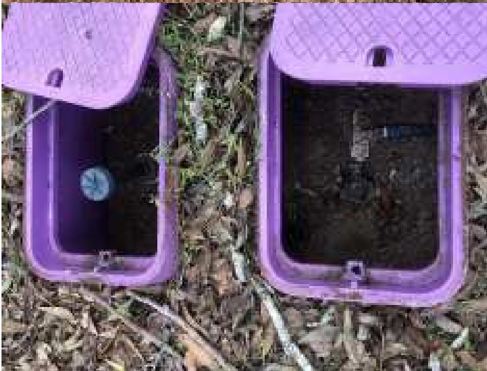
Photograph 11. View of flush valves and vacuum release valves in irrigation boxes.
