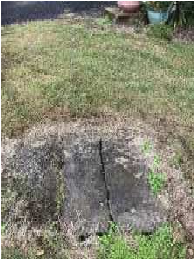
Photograph 2. Smaller swimming pool amenities septic tank (T2) (PW6).
