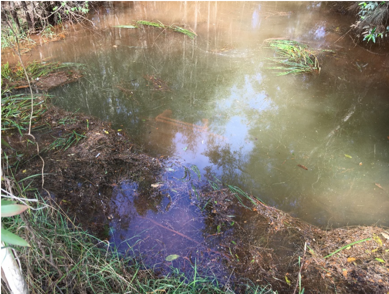
Broken Floodgate that can't be accessed or manually operated on Goodwood Street which allows water from Edwards Creek to drain back to proposed site.
