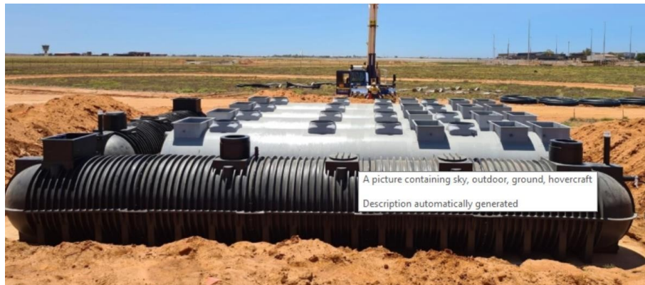
Figure 2 – Sample of Exposed Incomplete Packaged Treatment Plant Installation
