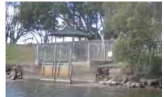
There are two pumping stations along the levee wall within the study area.
