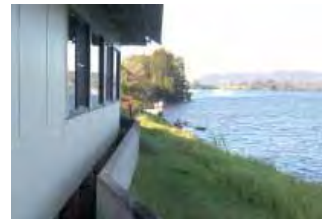
The levee wall is within private property in many instances, however this is a Council maintained asset.
