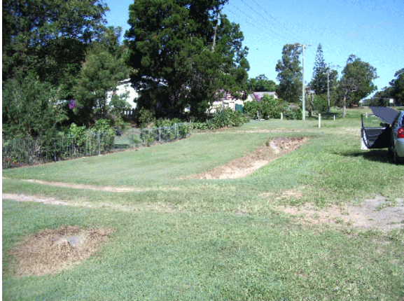
Photo 15: Typical area where ponding of local runoff will occur
