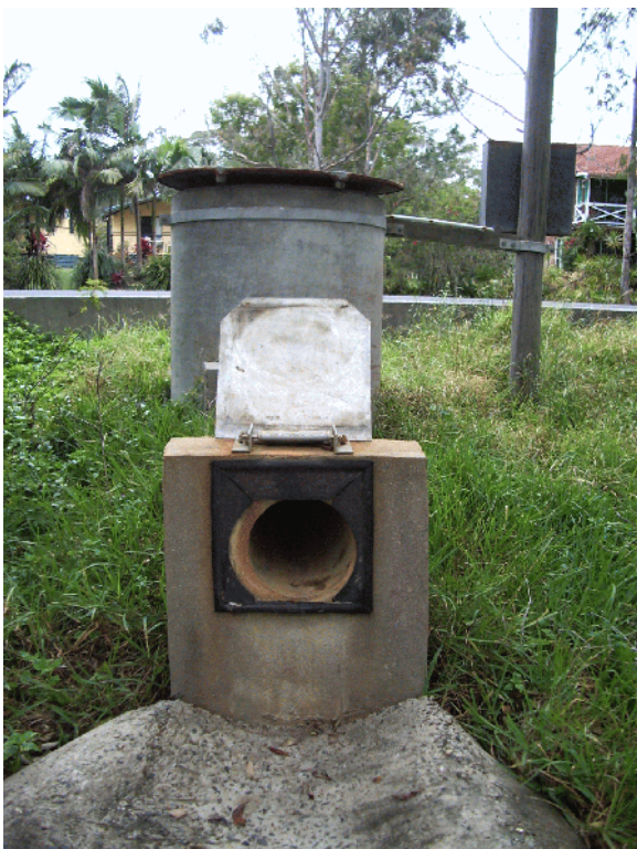
Photo 11: Pump within concrete levee system
